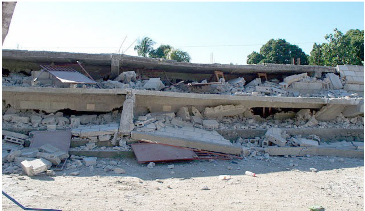
Sixteen out of 22 classrooms at Macombre Academy were destroyed.
